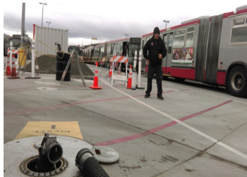
Figure 15. SMTA's underground RD tanks
