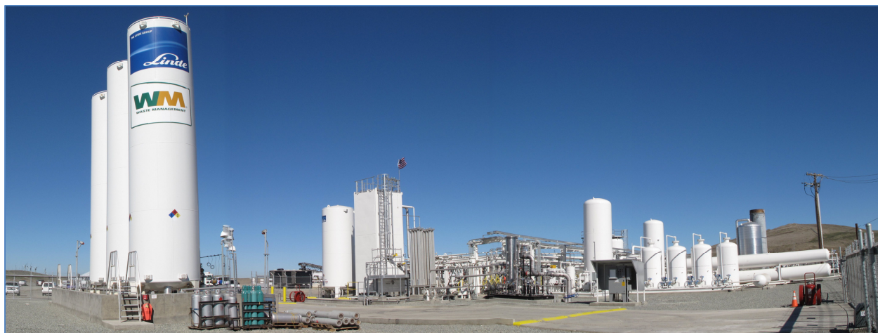
Figure 15 – Altamont LFG-to-LNG Facility
